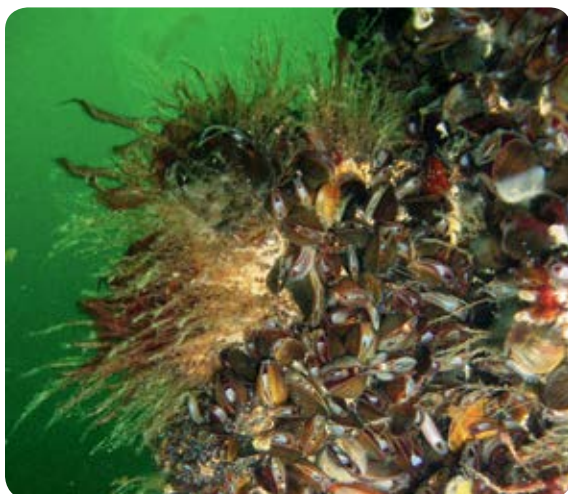
Figure 4: Fouling on wind mill foundations (photo: Mathias Andersson/Azote).
